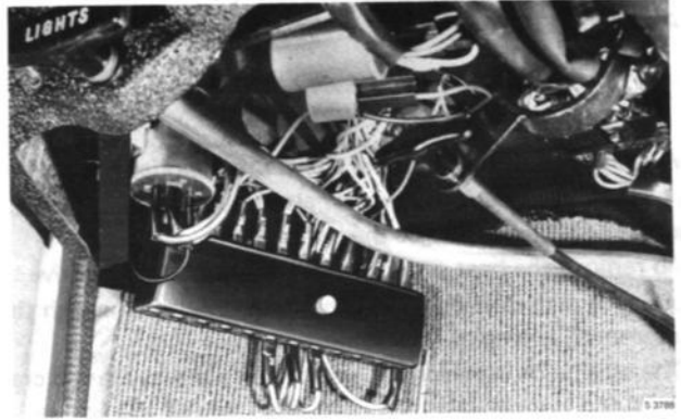
FUSE BOX UNDER INSTRUMENT PANEL
